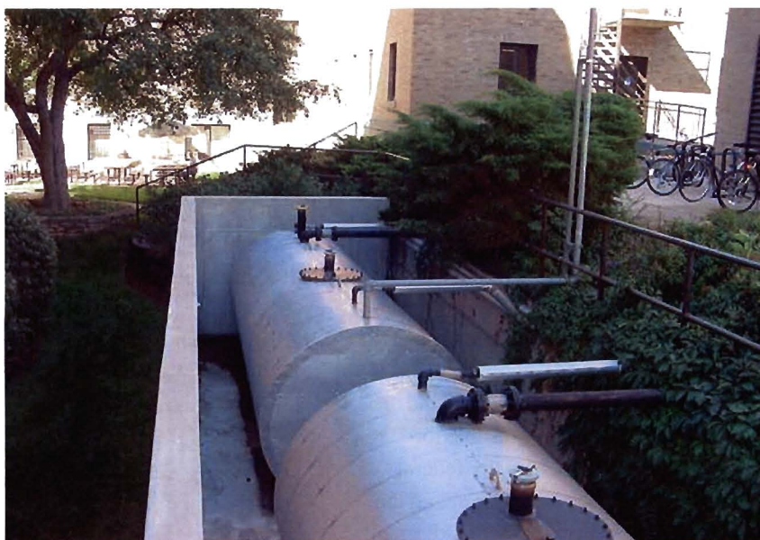
Aboveground fuel storage tank
