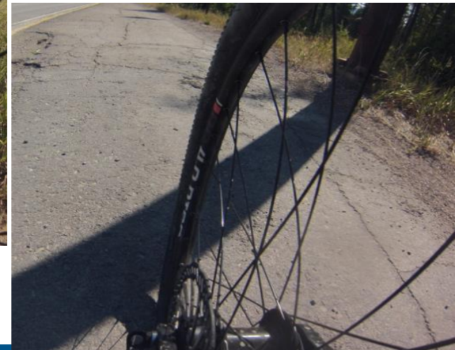
Paths in Poor Condition
