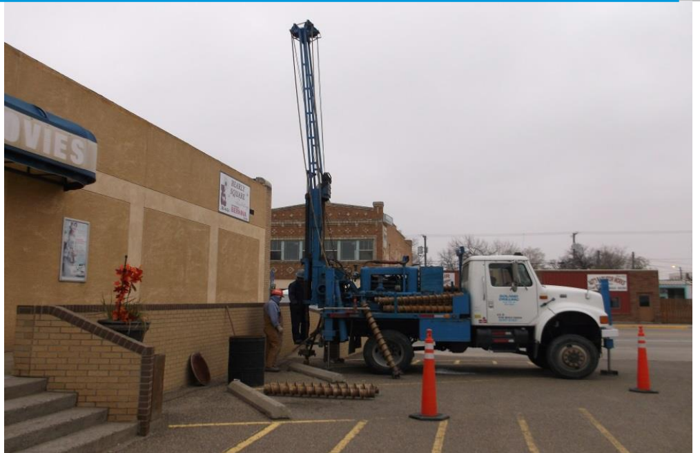
Installation of soil vapor extraction well at Former Roxy's Cleaners in Havre, MT
