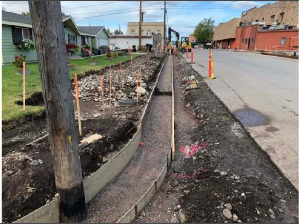
Photo #3 Curb and gutter forming on the south side of 6 th Street Sidewalk Improvements
