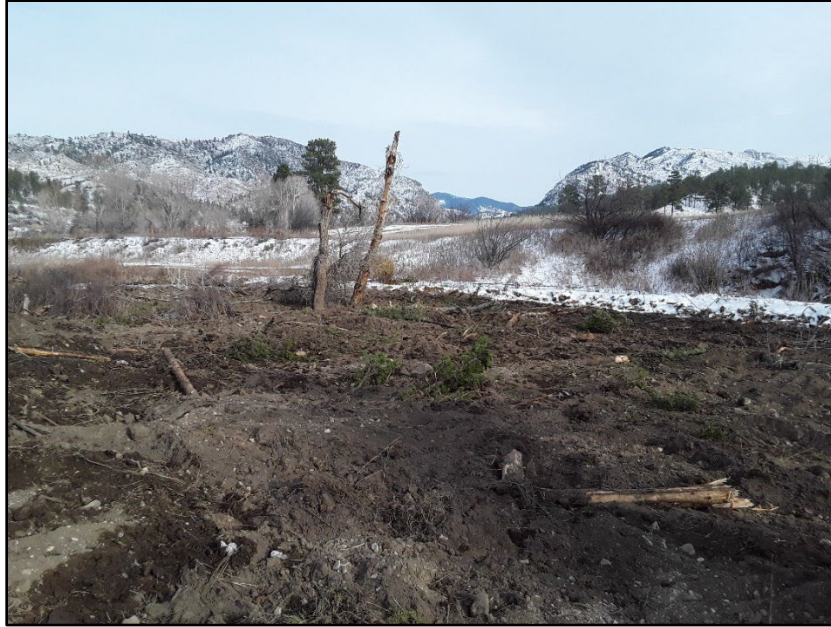
Figure 9. Completed channel and floodplain construction. The work incorporated juniper limbs buried category 2 wood to amend the soil and willow trenches were placed perpendicular to the channel. Wildlife snag pods were placed to create vertical structure inviting cavity nesters.
