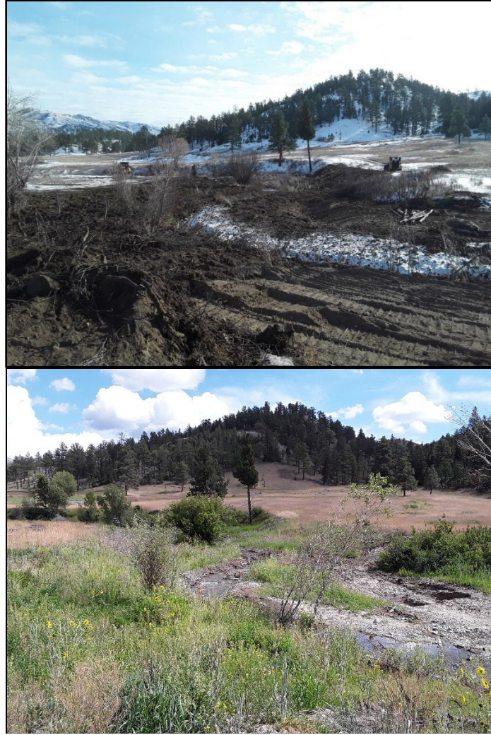
Figure 7 and 8 . View of Station 72+50 during construction looking upstream. Approximately 4,700 CY of net earthen material were moved to the repository, 9,400 CY were used to plug the old channel, creating a newly expanded and connected floodplain. Bottom picture Station 72+50 July 2023, 7 months post construction.
