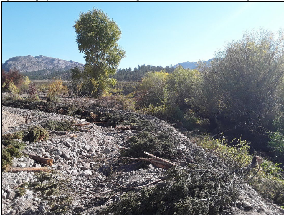
Figure 5. Channel construction at the top of the project area Station 53+00. Newly constructed channel was raised relative to the old channel (right) to increase floodplain connection and restore floodplain elevations to historic levels.
