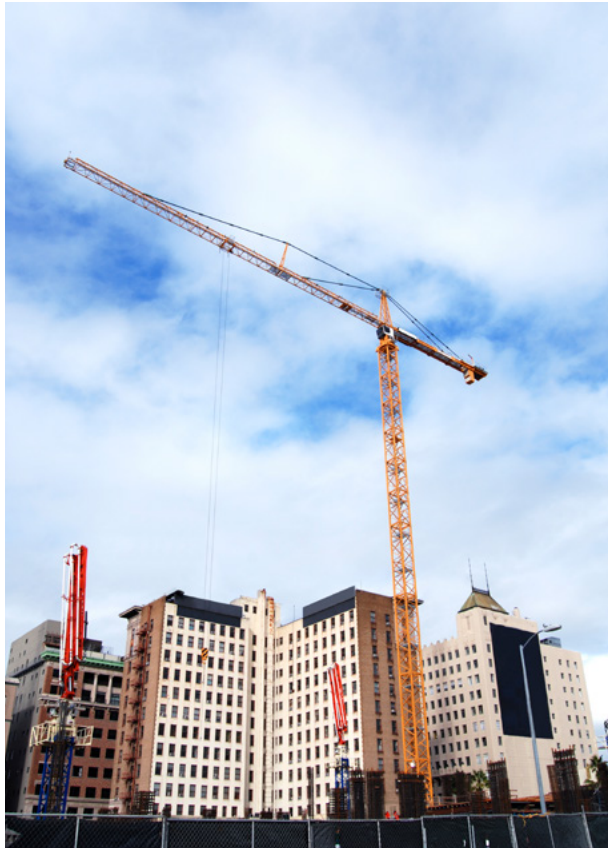
Construction underway in California, where officials require localities to submit annual reports showing progress toward state-determined housing production targets. Credit: rappensuncle via iStock/Getty Images Plus.
