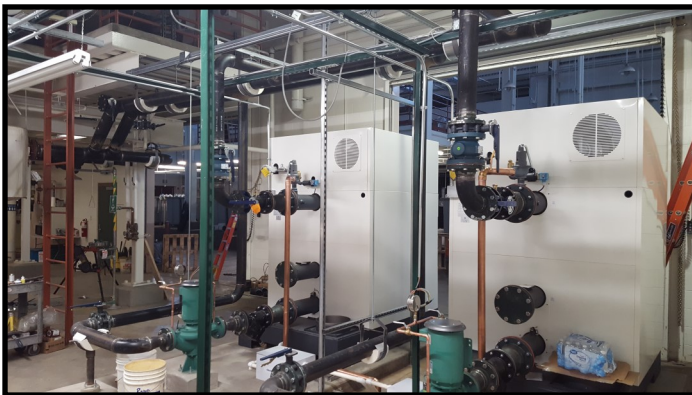
Photo 1: Twin 1-Million BTU Boilers
