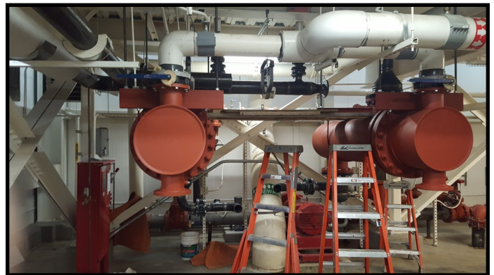
Photo 2: Twin "Tube-in-Shell" Heat Exchangers
