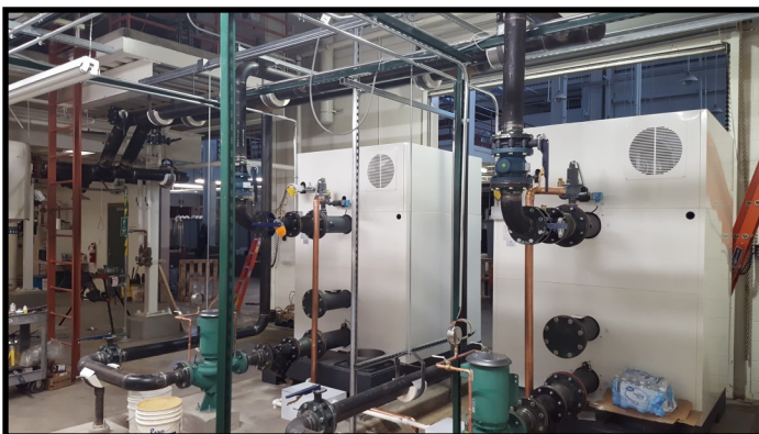
Photo 1: Twin 1-Million BTU Boilers
