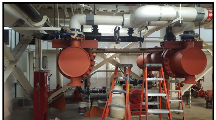
Photo 2: Twin "Tube-in-Shell" Heat Exchangers
