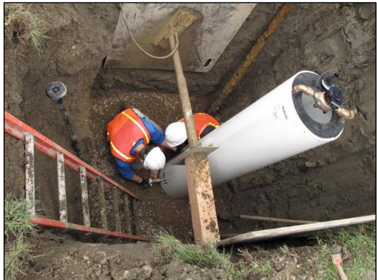
Renewable Resource Grant to Nashua to connect the town to the Fort Peck - Dry Prairie regional drinking water system
